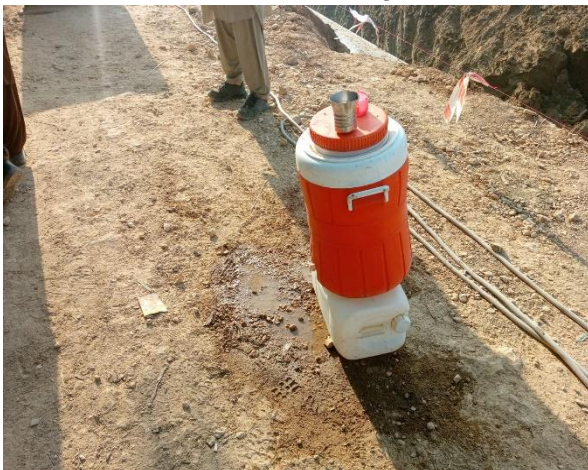
The fresh drinking water was provided to the labor
